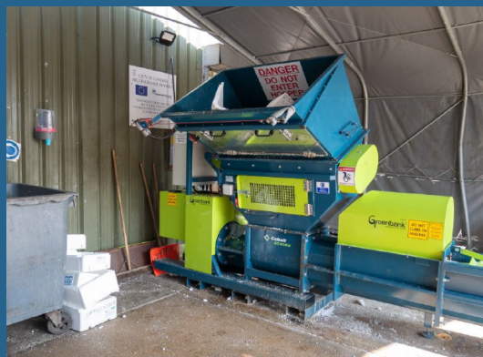
EPS recycling machine at Billingsgate Fish Market in London (photo: Repak)
